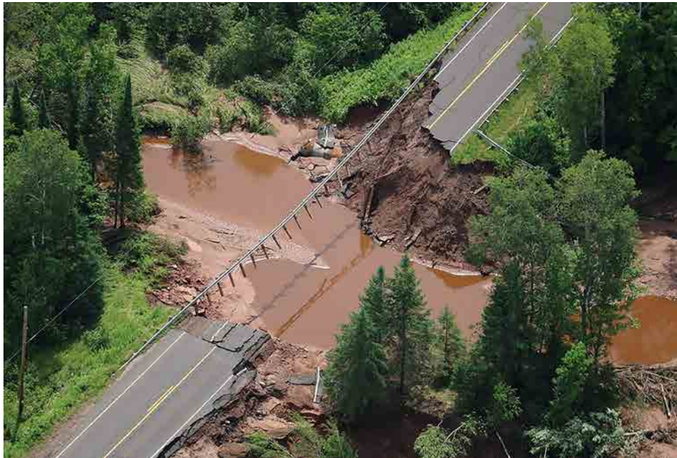
A WisContext report on climate change featured this bridge in Bayfield County overcome by flooding at the end of summer. (CREDIT: Wisconsin Emergency Management)
