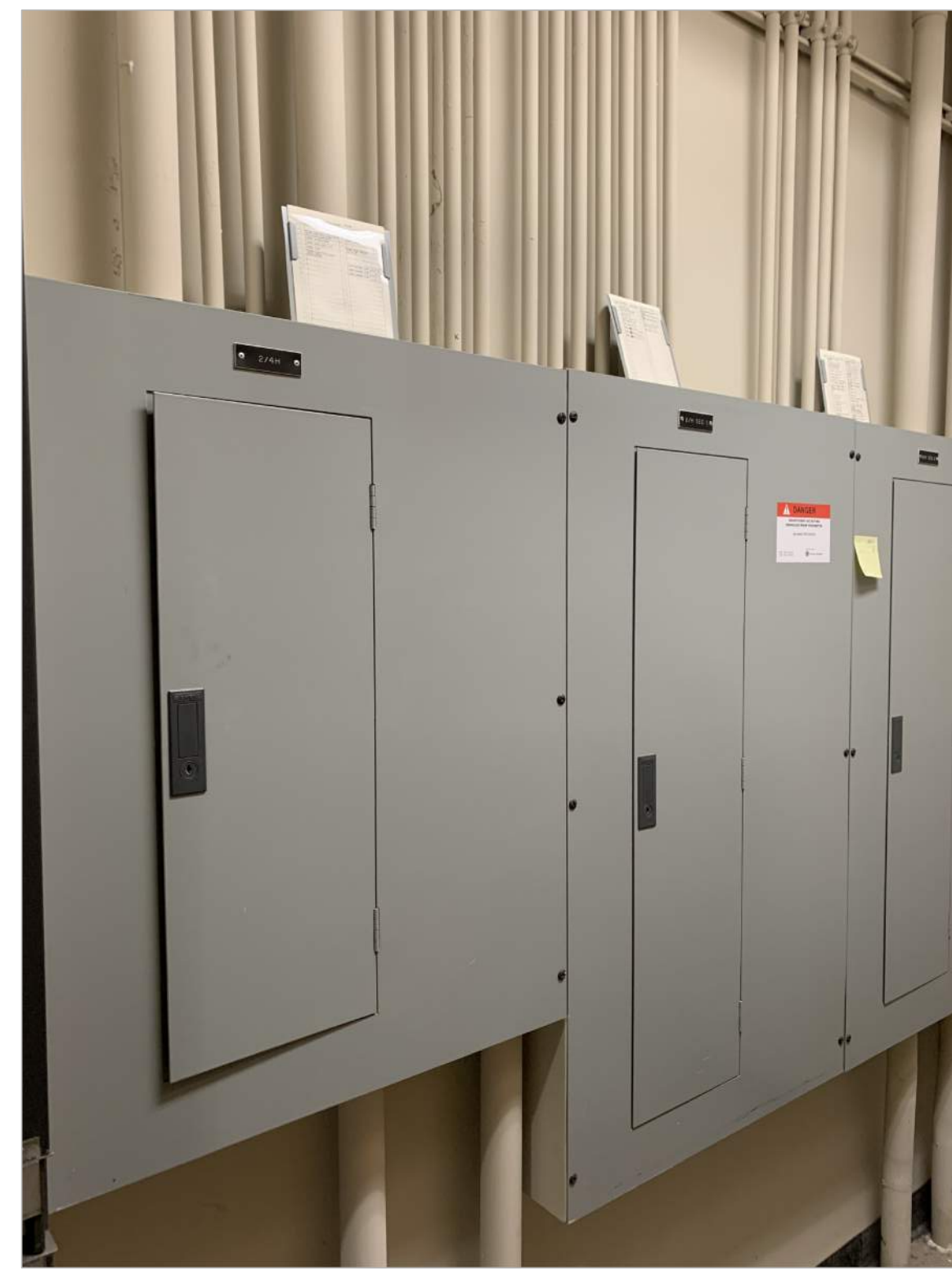
3 EXISTING 2ND FLOOR PANELS 2/4H, 2/4H SEC 1, 2/4H SEC 2 PHOTO NO SCALE
