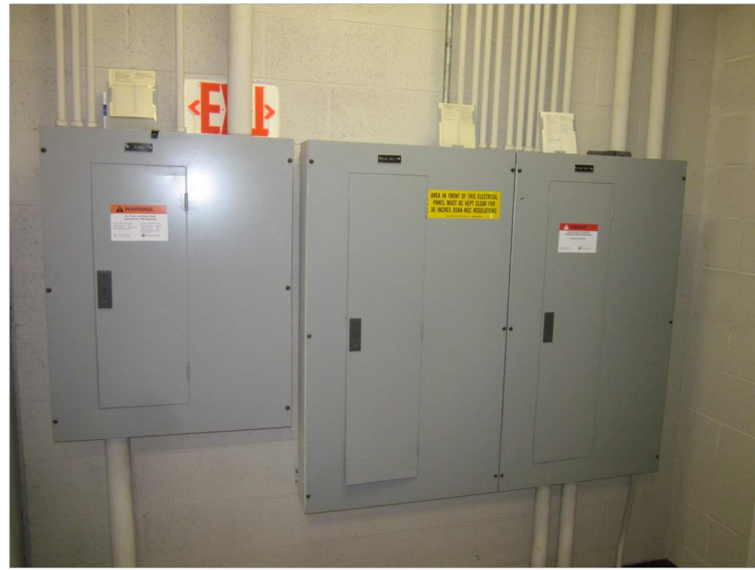
3 EXISTING 5TH FLOOR PANELS 5/4Q, 5/Q SEC 2, 5/Q SEC 1 PHOTO NO SCALE
