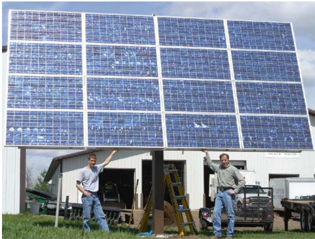
Steiner Plumbing & Electric PV Project, River Falls
