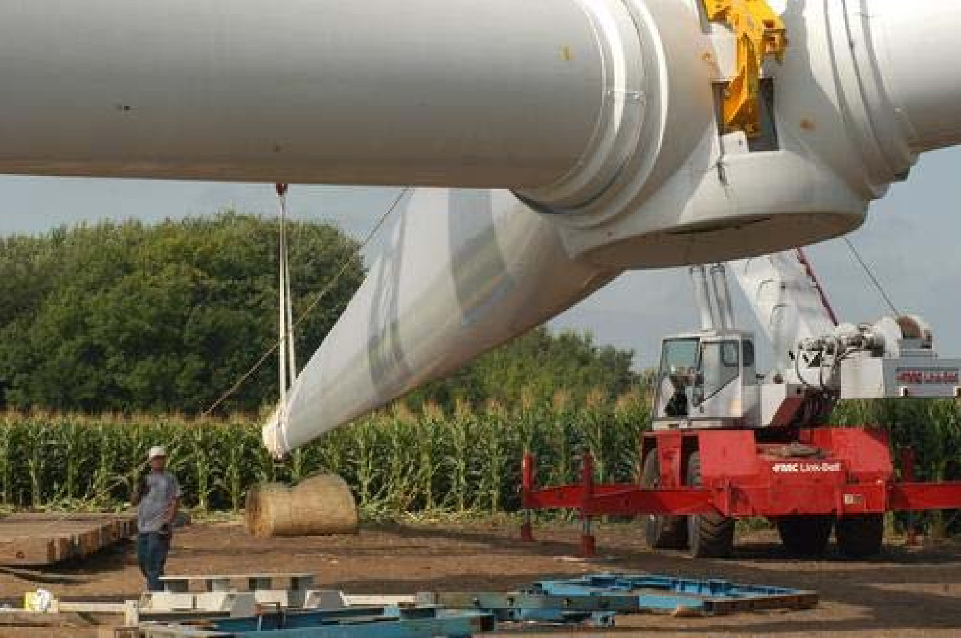
Turbine and three 135 foot blades atop a 230 foot steel tower.
